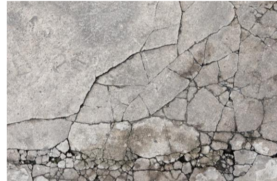
Figure 3: Crumbling concrete driveway [3]
