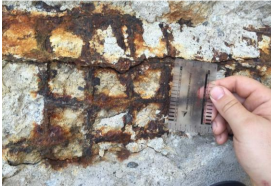
Figure 2: Concrete chloride attack [2]
